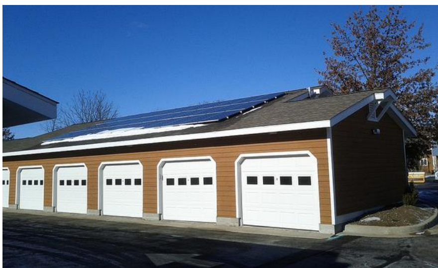
Figura 7 - Painéis solares – Great Oak Cohousing
