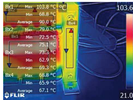
Figure 5.1 Thermal image of the transformer after 200 minutes.
