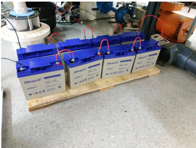
Figure 4.10: Bank of batteries
