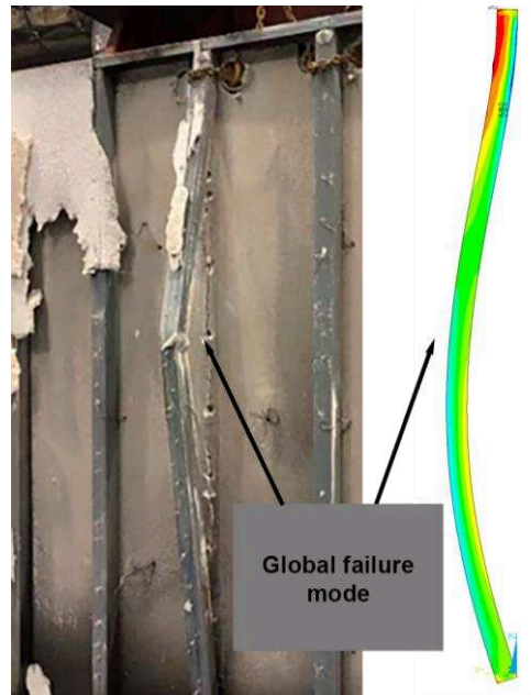
Figure 4.43 – Critical failure modes of stud 4 from fire test specimen [9] and stud 4 at failure time from FEM.
